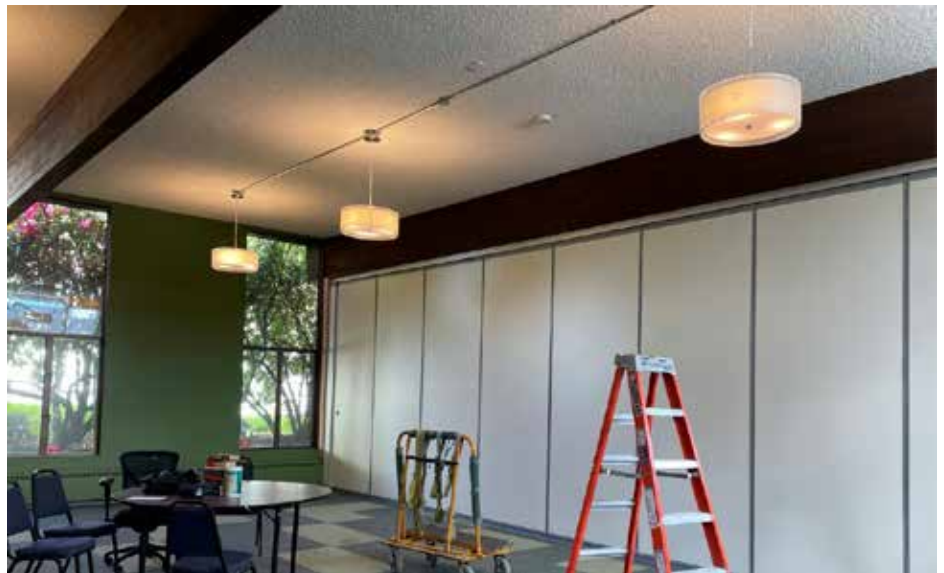
Fellowship Hall Operable Partition
