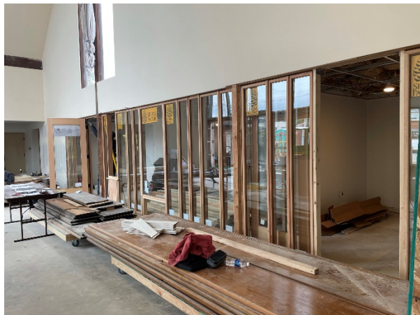
Narthex / Admin Storefront System (Open areas will be filled with reclaimed pew wood and intermittent glass panels will receive an opaque film)
